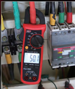
High voltage (600V) frequency measurement
