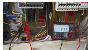
Automatic Voltage Measurement
